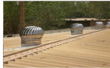
Hot air exhaust via mechanical turbines
