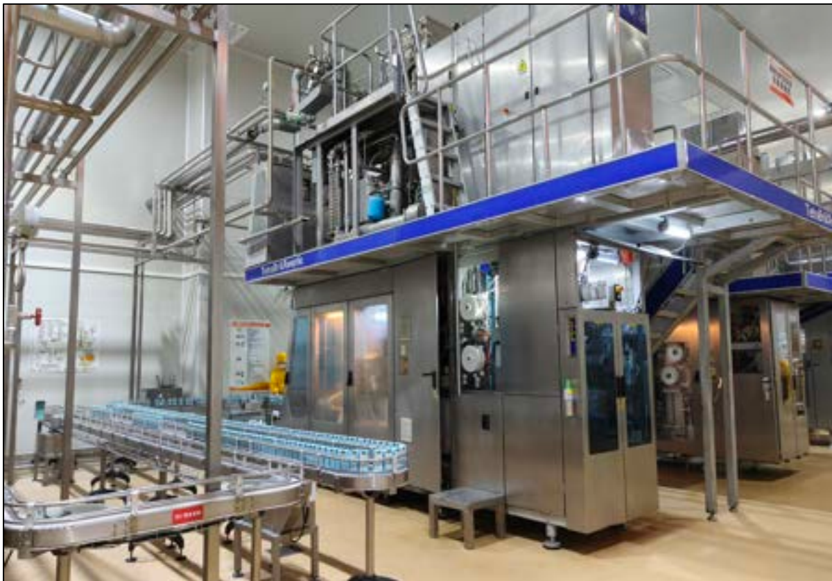
Figure 17. Aseptic filling and packaging machine
