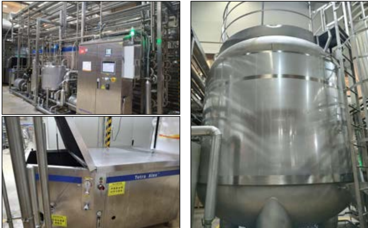
Figure 15. Ultra-high-temperature sterilizer, homogenizer, and aseptic tank
