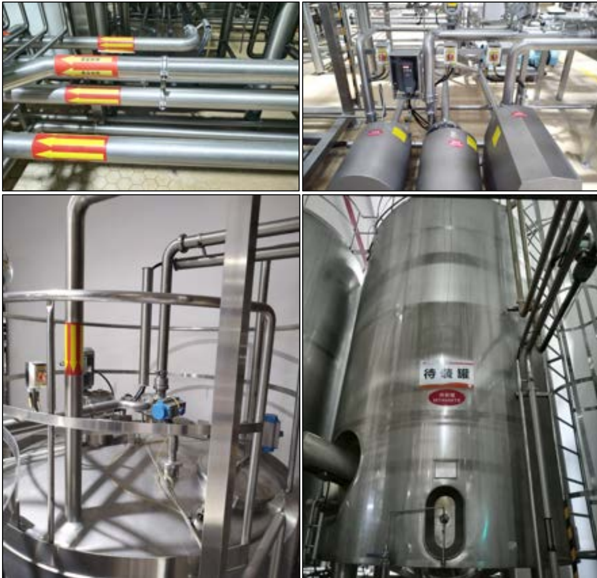
Figure 14. Materials pipelines (with arrows), pumps and semifinished storage tank
