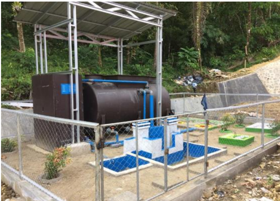
Figure 19: Waste water treatment facility at Puskesmas Hilisataro, Nias Selatan, North Sumatra. Credit: Rahmi, the MoH
