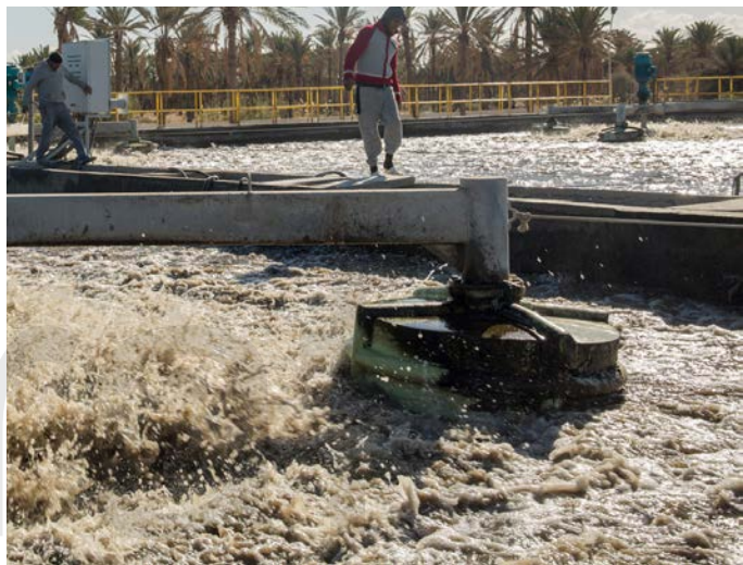
Wastewater treatment plant, Tunisia. © WHO/Diego Rodriguez.
